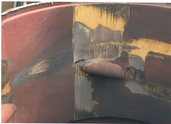
Baffle plate for wet steam in experimental boiler of KEMA.(photo KEMA). (2.133)
